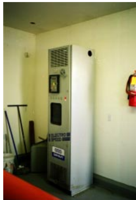
Figure 6. Exterior of the variable speed drive.
