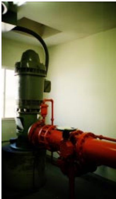
Figure 5. Well No. 4 Pump
