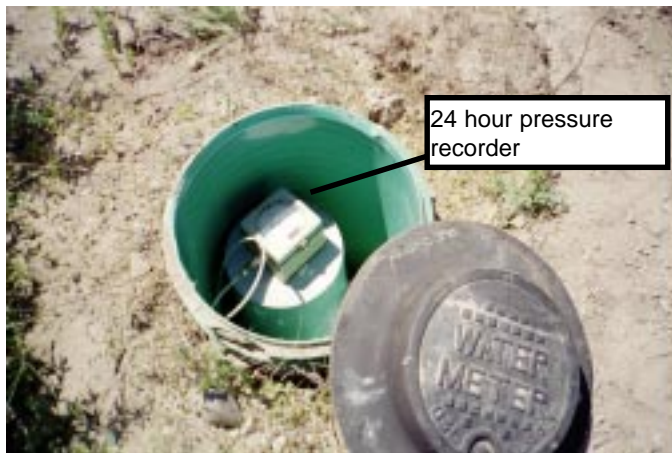
Figure 14. 24-hour continuous pressure recorder installed in meter box.
