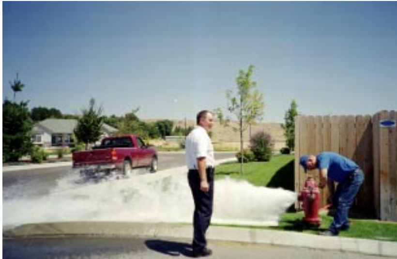
Figure 19. Norman Revels of Eagle Water Company and Kurt McClenny of the Eagle Fire District perform a fire flow test on a hydrant at the Eagle Springs Clubhouse on July 27, 2000.
